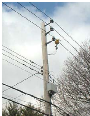
Utility pole mounted Ambient Corp BPL equipment (photo by N2YGK).
